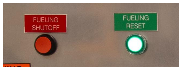
Fig. 1.2.1 - FUELING SHUTOFF and FUELING RESET Buttons
