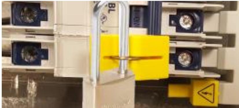
Fig. 3.3.5 – Breaker Locked Out with LOCKOUT Adapter
